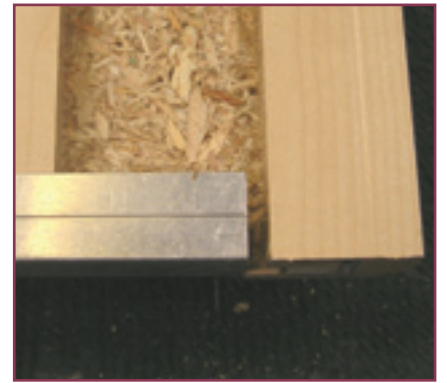
9. Using a rubber mallet, gently tap on the stile to the side of the panel, aligning the bottom of the stile with the bottom aluminium rail. (Use a small off cut as a guide).
