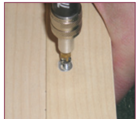
12. Fix by using 6 1/2" counter sunk screws so they lay flush at the back of the stiles. Repeat the other side
