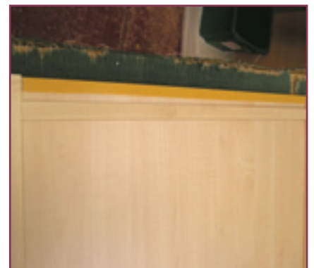
21. Cut the 25mm Top rail trim. Remove the yellow part of the double-sided tape already on the top aluminium rail and stick down, applying plenty of pressure.
